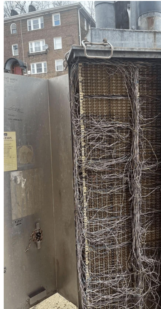
The inside of a cross-connect cabinet in a metro area
